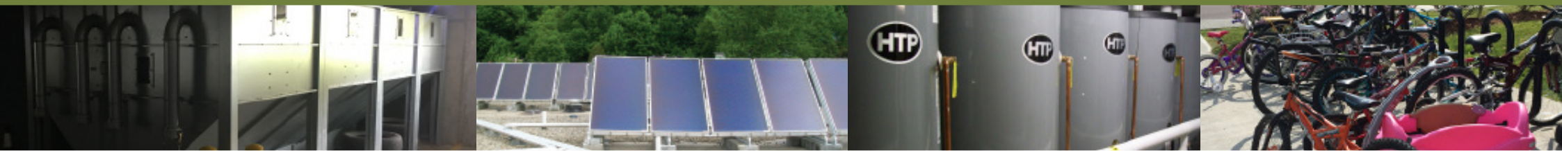
Left to right: River Station Apartments in Montpelier is heated with a wood pellet boiler; solar panels on the building's roof provide the energy needed to heat the hot water for the building; hot water tanks hold located in the basement of River Station; bike racks at South Main Apartments in Waterbury encourage our residents to travel "green".
